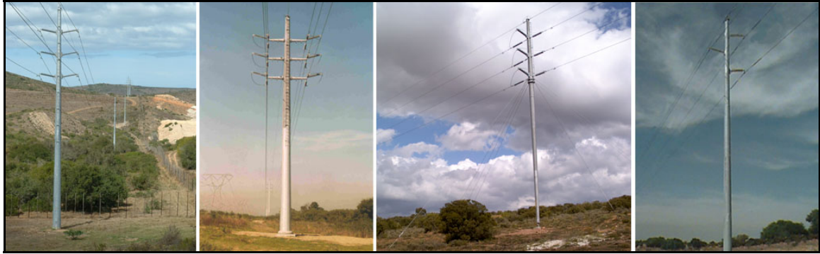
Figure 24: Examples of monopole distribution power line towers.
